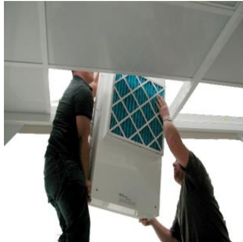
Figure 6: FFU rotated 90° and lowered completely from ceiling grid
